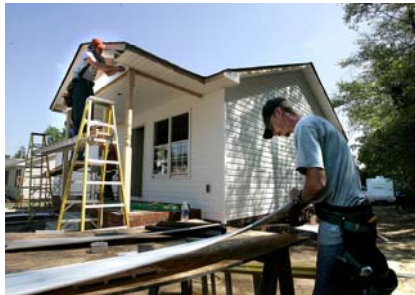
PHOTO COURTESY OF SHELBY STAR Jason Wright, on ladder, and Matthew Hyland work in front of Blitz house.
